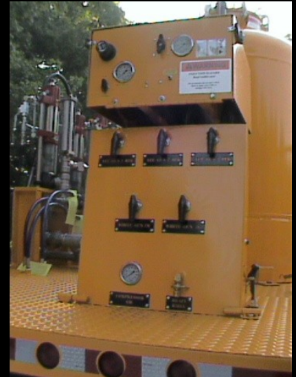
Control console with panel-mounted valves
